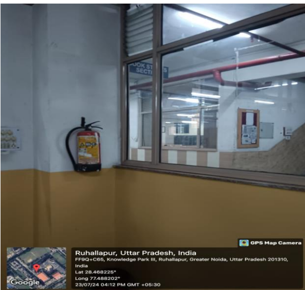
FIRE FIGHTING EQUIPMENT
